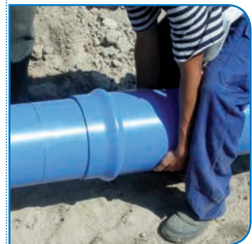
Align the pipe and place the spigot end inside the socket or bell.
